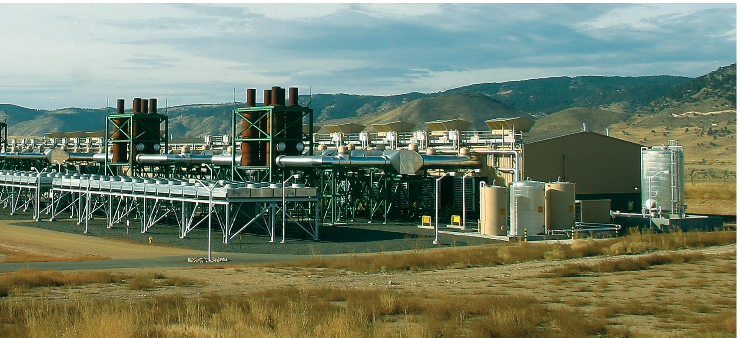
Fig. 1. Plains End power station in Colorado. This facility with a combined output of 231 MW is an example of a modern gas-fired commercial power plant based on gas engines. It has been in operation since 2001 (section I) and 2006 (section II), providing a way to balance unstable wind power output.
