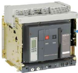
600 Volt Insulated Case Breaker Squared D Masterpact NW
