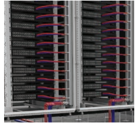
Rack manifold to manage liquid distribution
