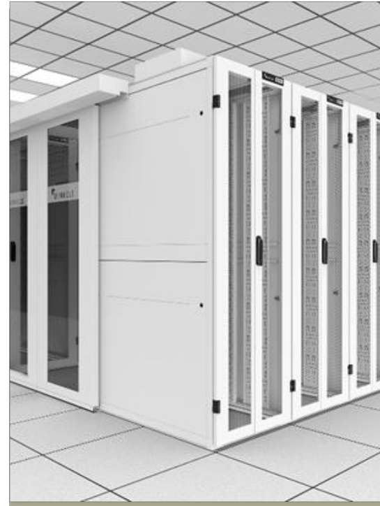
Datacenter cold aisle containment
