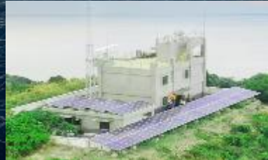
Solar access in CO rooms @Zhuhai 100% green power
