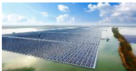
Floating solar plant 60MW @Huaibei, Anhui
